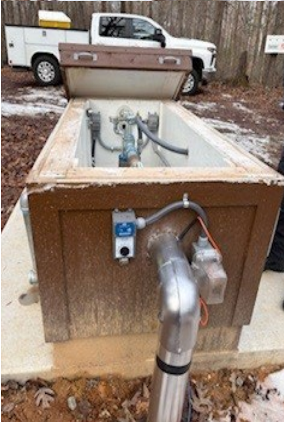
Figure 6 Old Mill Trace Well Pump
