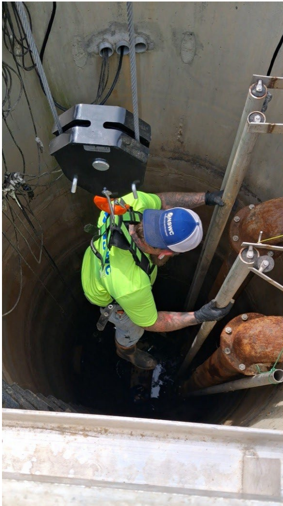
Figure 2 Briar Chapel 5 Day Pond Lift Station
