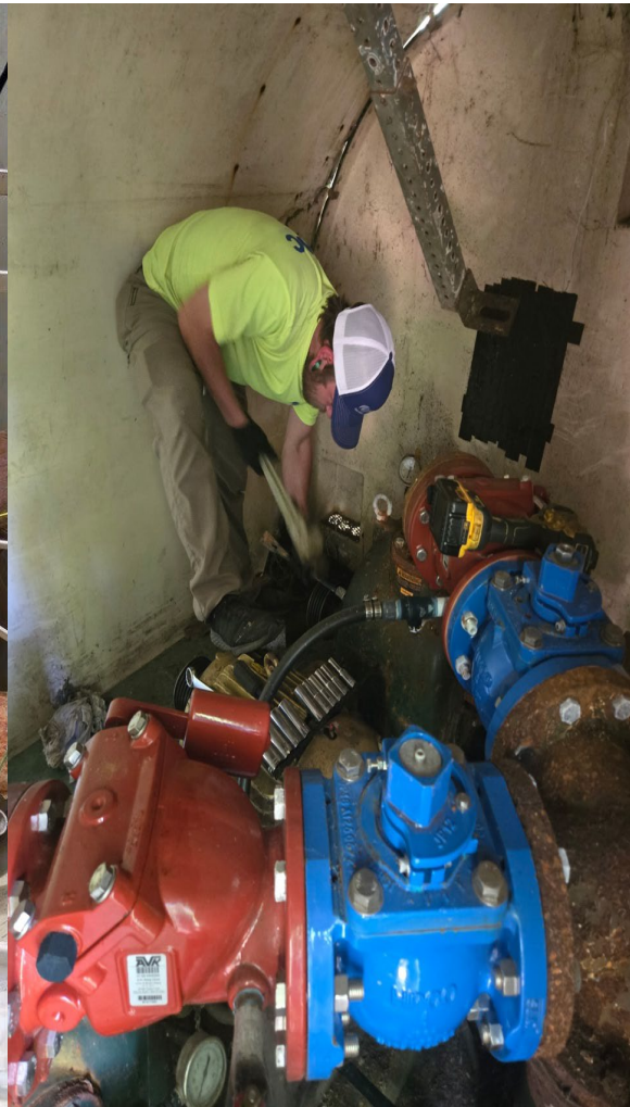
Figure 3 Bingham Woods Lift Station
